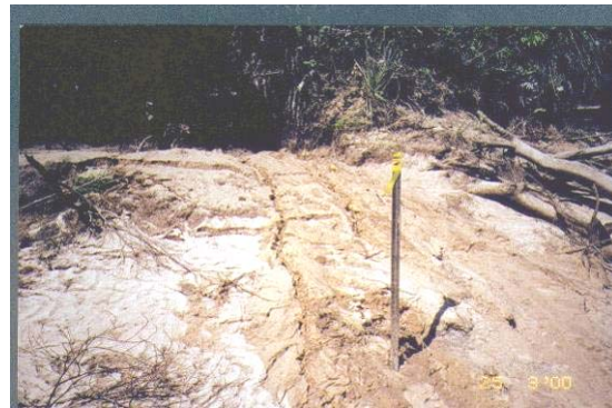
site 2K March 2000 – note rilling and angle of tree stump in left side of photos.
