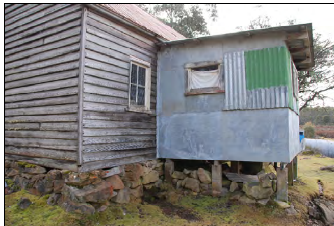
Photo 20: corrugated iron patching.
