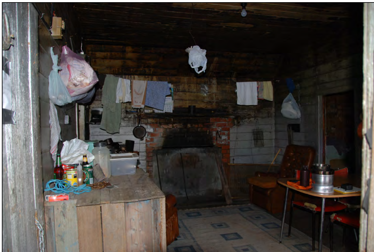
Photo 30: Central living space and fireplace, looking from entrance porch. Note soot residue on west wall and ceiling.
