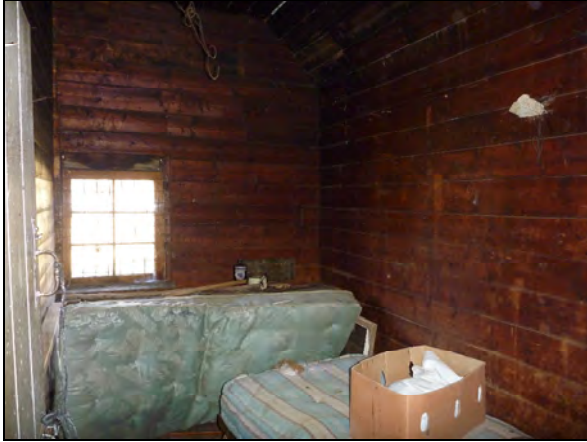
Photo 37: south west room, looking south with bed, window and bench beneath window.
