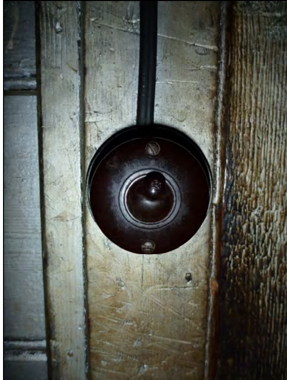
Photo 24: typical Bakelite electrical fitting.
