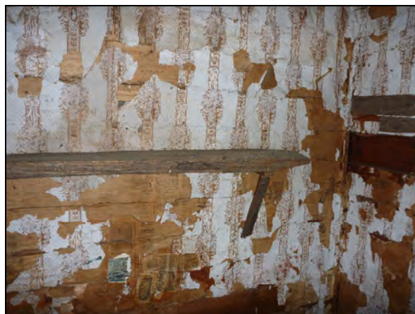
Photo 32: south east room, with bench, newspaper and wallpaper remnants.
