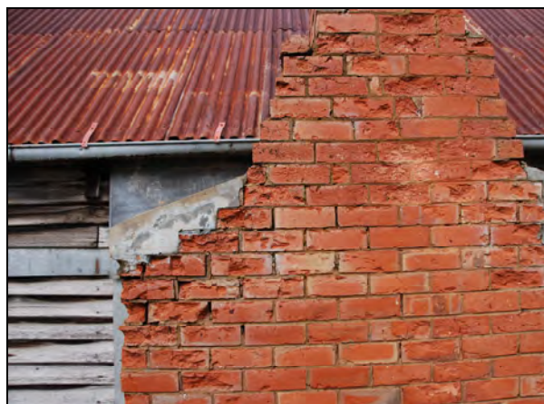
Photo 22: 2004 cement repairs and missing mortar.
