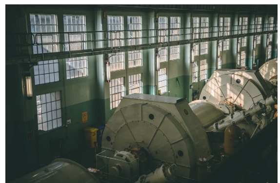
Figure 29: Turbines at Tarraleah Power Station
